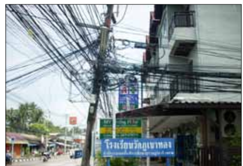
The Thai way of electrical wiring ...
