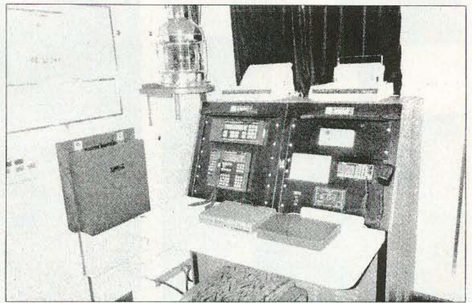
Photo D. The radio communications system on the bridge of the Big Red Boat III was well maintained.
