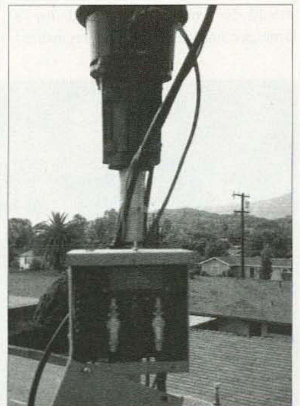
Photo B. The electrical box with the two preamps installed in it.
