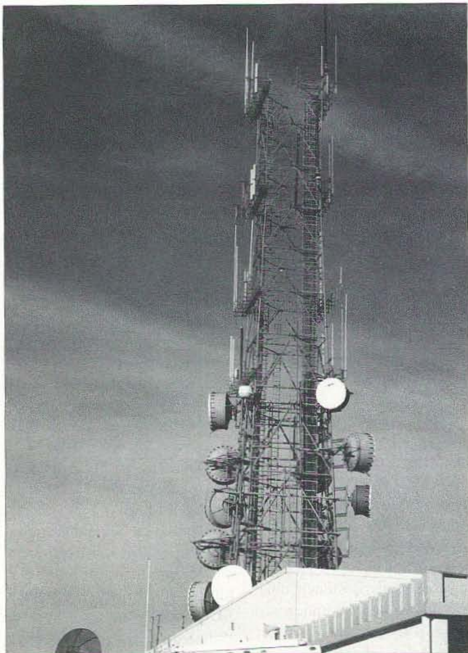
Photo A. Transmitters everywhere! With all the communications sites like this one, plus RF-emitting devices in almost every home and business, it's no wonder that unintentional interference is a growing problem.
