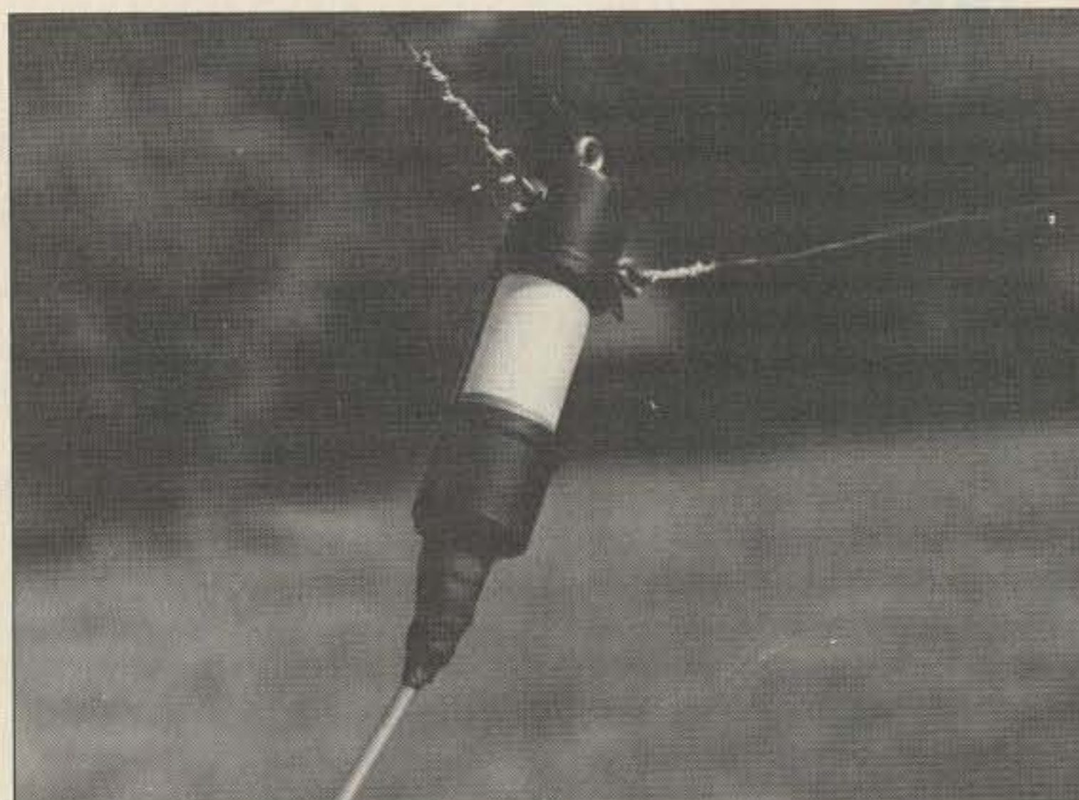
Photo A. One of the baluns on my antenna system. Note coax sealer and the soldered connection to the balun and antenna wire.
