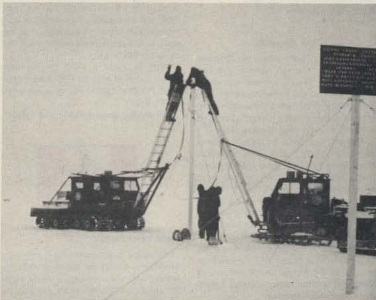
The last connection is made on the 26-mile-long ULF dipole antenna at Siple Station. Four thousand feet of salt-free ice (accumulated snow) beneath the antenna provides insulation from earth ground.
