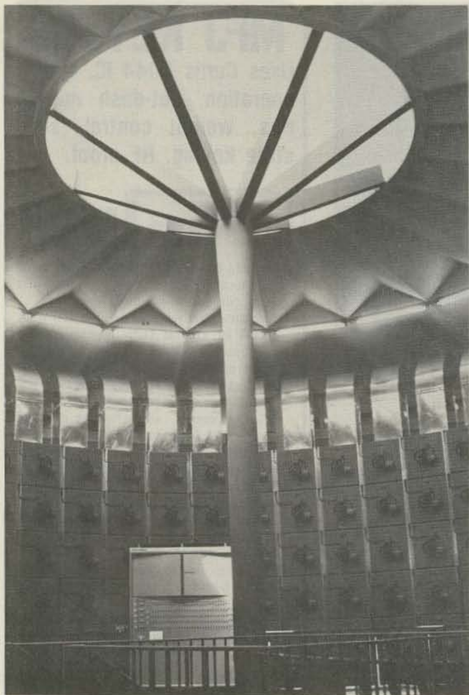
Antenna side-switching hut showing a portion of antenna routing system. Each "square" is a motor-driven switch.
