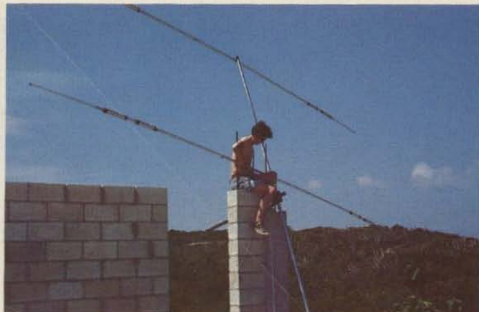
A partially-completed cinder-block wall provided a sturdy support for our tribander. Here, Tim prepares to hoist the antenna into place on a protruding piece of reinforcing rod.
