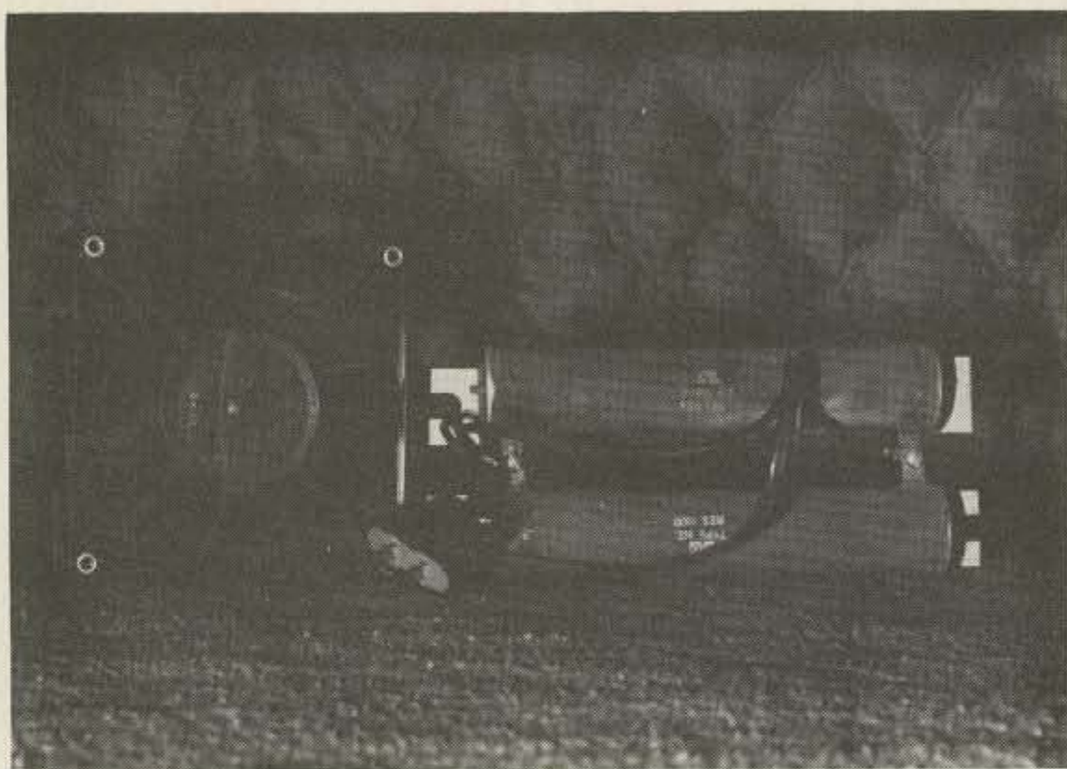
Photo E. The unclassy method of slowing down a fast, noisy fan, with power resistors. These two units need to be mounted in a well-insulated box, or be replaced by a much more elegant capacitor.
