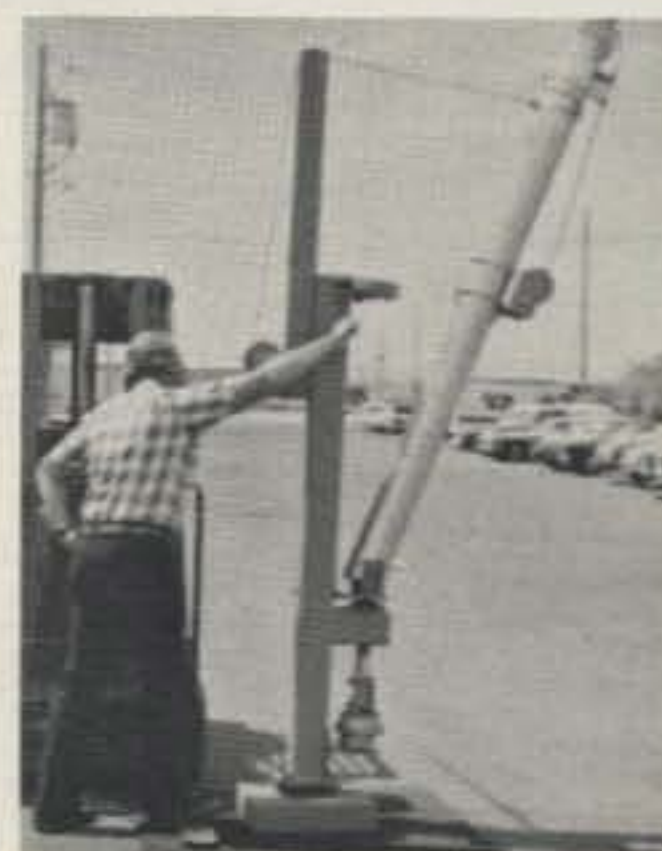
Tilting the tower over is a one-man task with the Wilson bases.
