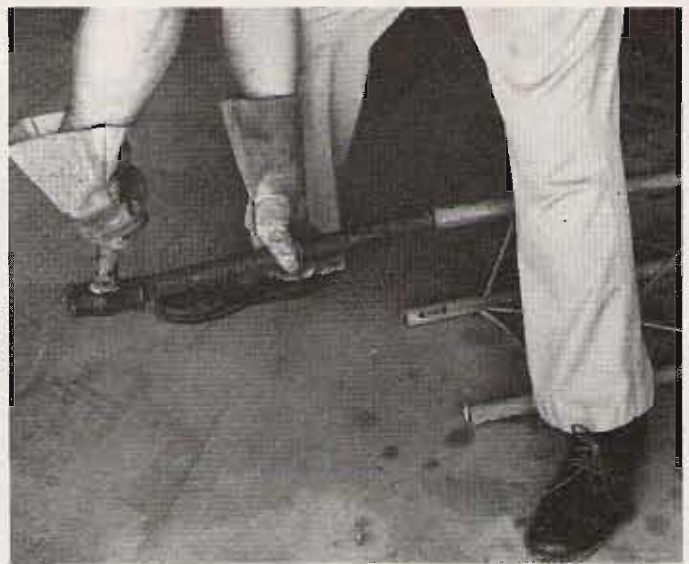
Photo F. Clearing excess galvanizing from the tower legs will make joining easier.
