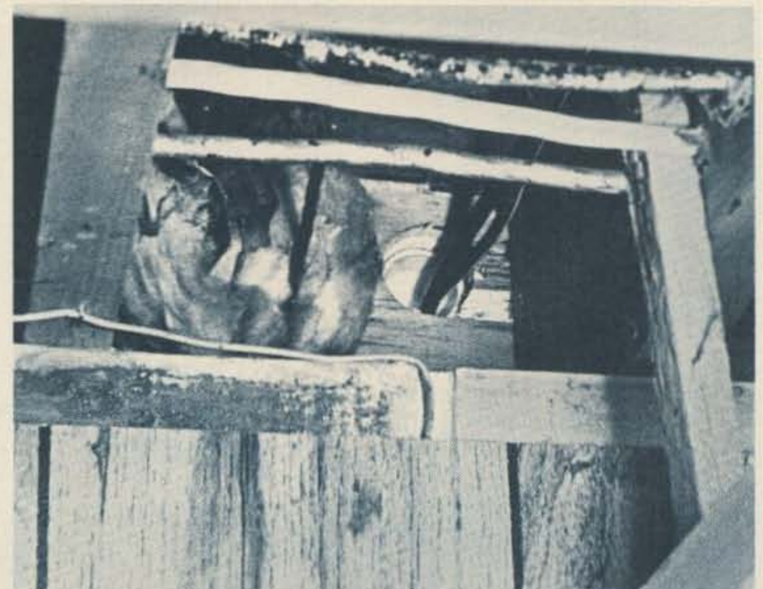
Inside-of-house view of the 90° elbow and the cables routed through it into the house.
