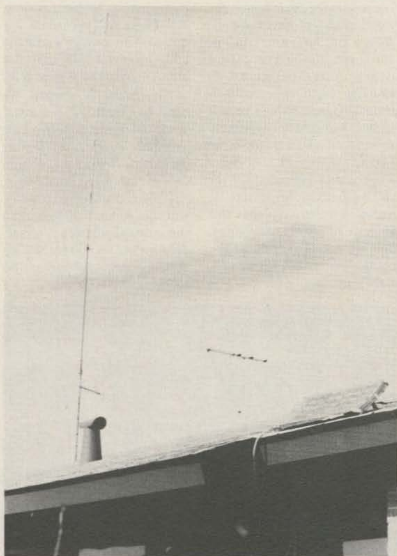
The multiconductor cable hanging from the left of the solar cell array is used to measure individual cell output, if desired.
